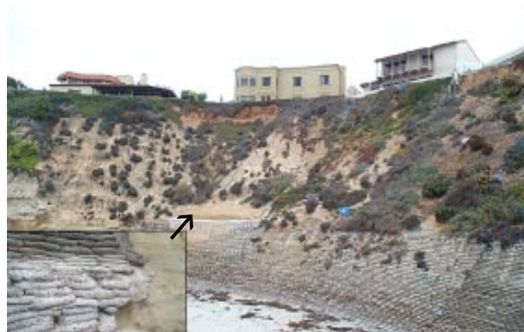
Concrete wall at bluff base in Solana Beach. Inset shows detail of wall failure, also visible in center of photo. Photo: Scott Ashford, UCSD
