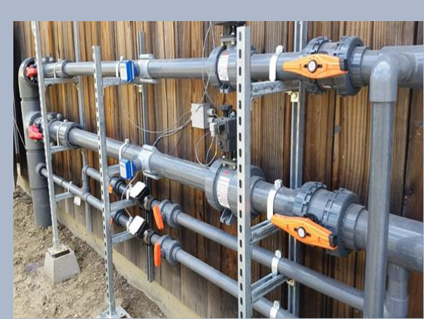
The control system of the pipe, at the pump house by Gallo's reservoir.
