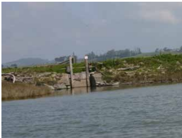
Many tidal sloughs are controlled by tidegates
