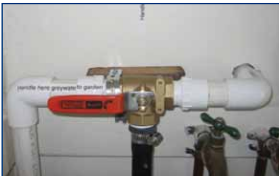
Close up of valve that switches graywater discharge from sewer line to graywater irrigation system.
