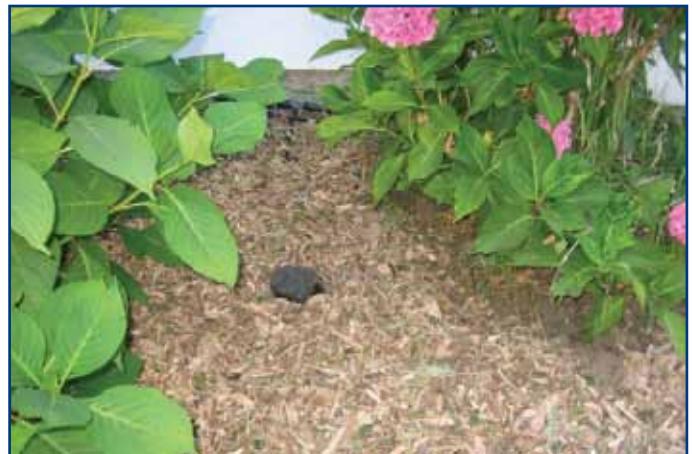
This subsurface outlet provides ornamental shrubs with graywater. Photo by Greywateraction.org .
