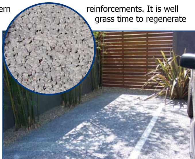
Close up of pervious concrete shows void spaces between the open-graded aggregate where water filters down.
