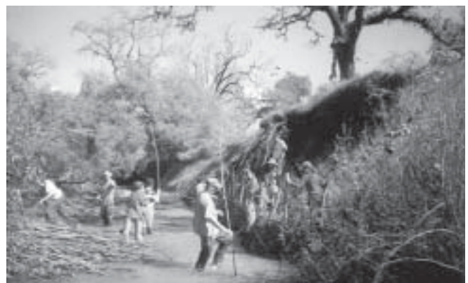
Restoration project to stabilize an eroding stream bank by constructing a willow wall and recontouring the slope of the creek bank.
