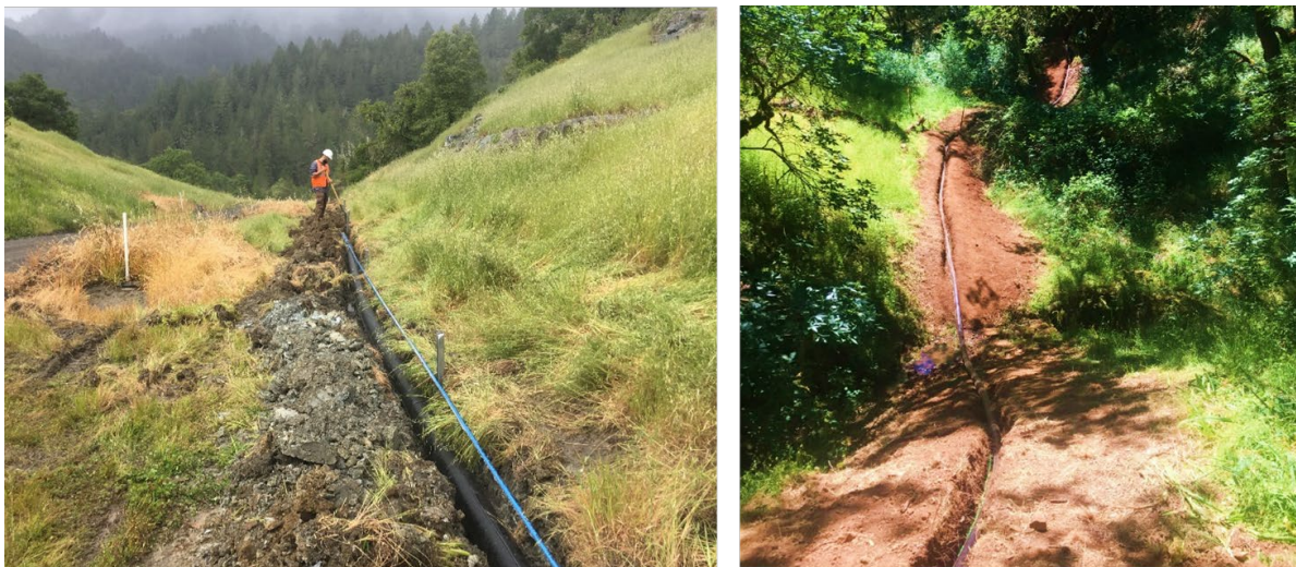
Figure 3. Installation of six-inch (pictured left) and three-inch (pictured right) HDPE pipe to carry water from the storage pond to the Porter Creek release points.
